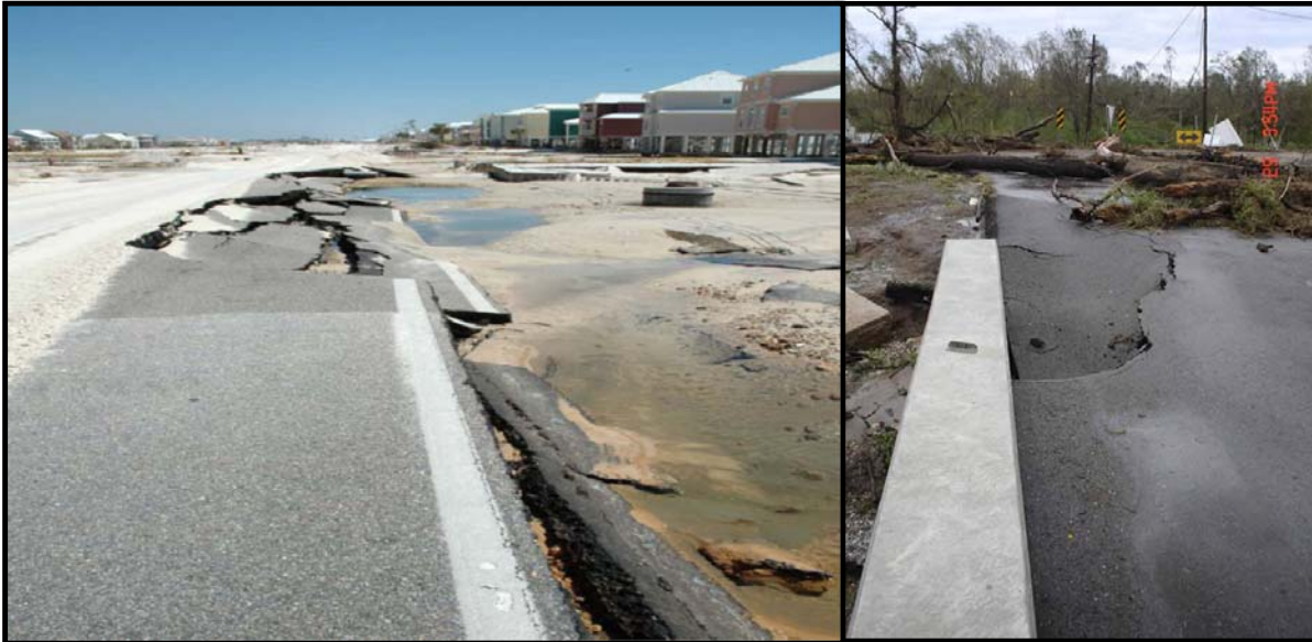
9 10 11 12 13 14 15 16 17 18 19 20 21 22 23 24 25 26 FIGURE 1 Examples of Damage-Passable Pavement Damage Post-Natural Disaster.
