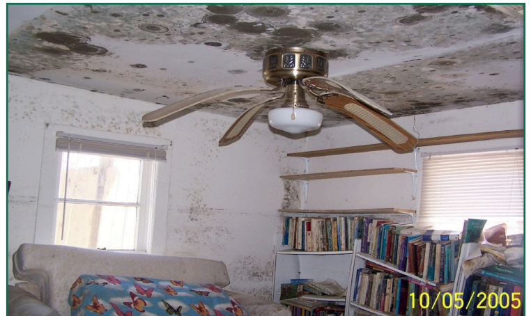
Mold growth inside a home after Hurricane Katrina in Gulfport, MS.
