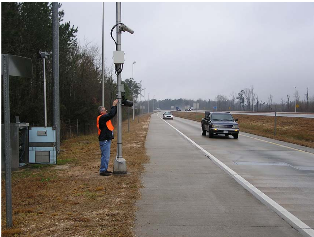
Figure 3. Installation and alignment of the PIPS ALPR camera.
