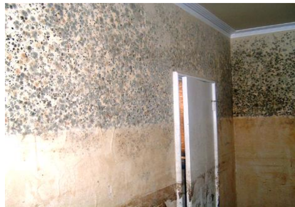
Mold growth can be very heavy as in New Orleans after Hurricane Katrina
