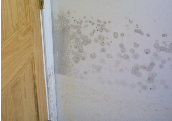
More typical mold growth is seen in the Tuskegee University test house.
