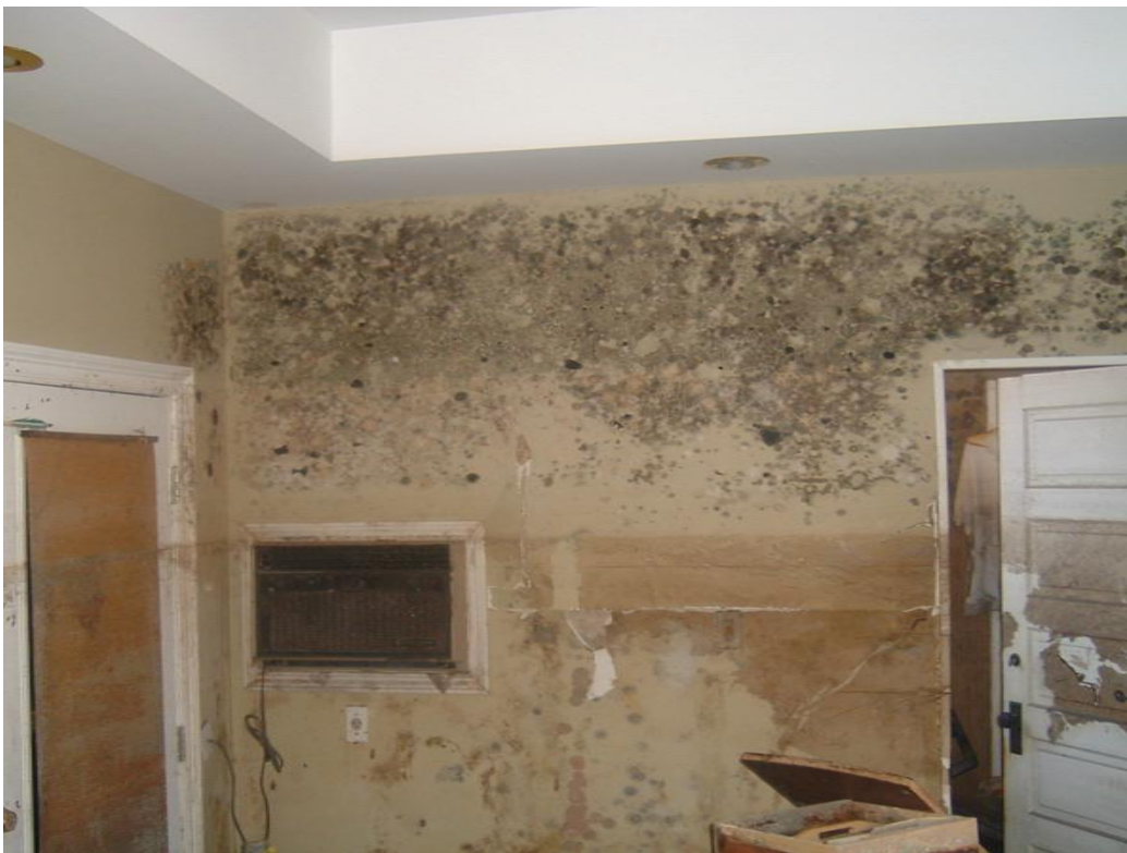
Figure 1. Significant mold growth occurred in a New Orleans, LA home after Hurricane Katrina and related the flooding
