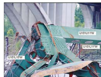
Figure 2 Damaged section of I-35 (www.enr.com)
