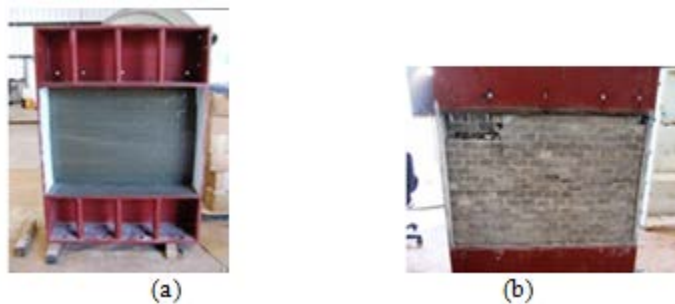
Figure 8: Wall #3 (a) Back view after the blast event (b) Front view after the blast event
