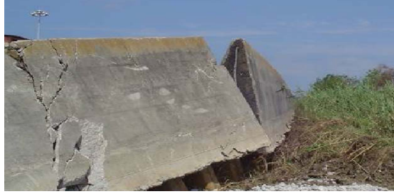
Fig2: Local Failure of one panel (IPET V-14-64)
