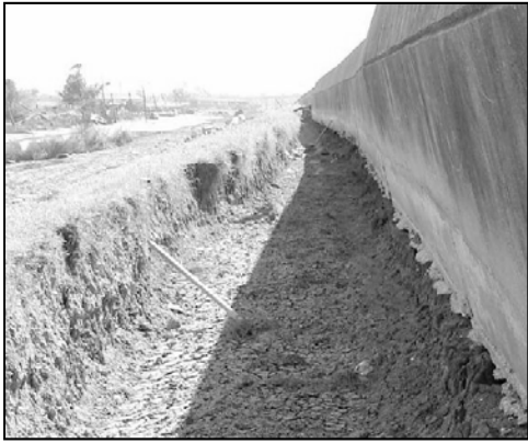
Fig. 1. Scouring caused by overtopping
