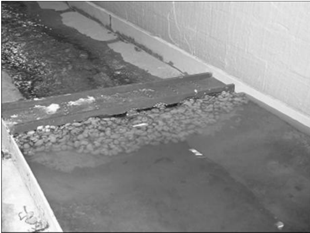
Fig. 4.6. Closure at Hammond Highway Bridge by using a combination of toe and transverse dumping for Cases 1 and 2 (looking south)
