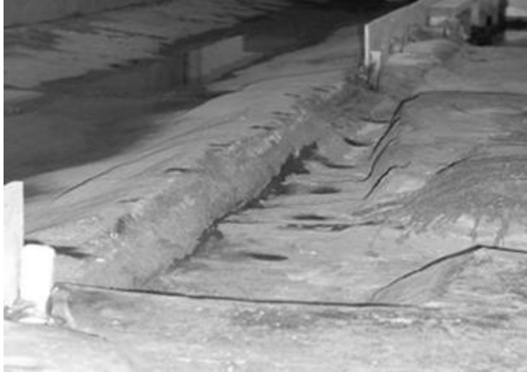
Fig. 1.3. The scour hole caused by landing slide and flood flow
